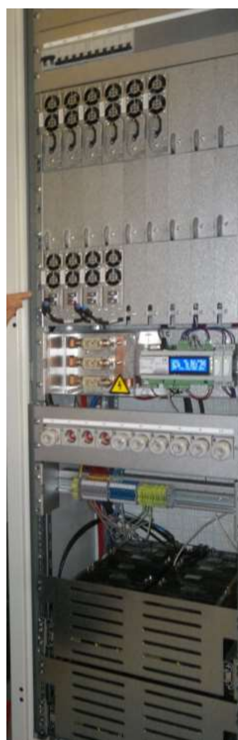
DC UPS & Batteries
